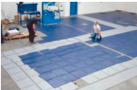
Pic 4. Split the pallet and spread the tiles across the floor prior to starting installation.
