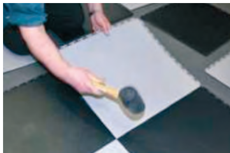
Pic 5. Don't force the tiles, offer up the corner of the tile and gently hammer the joints together.
